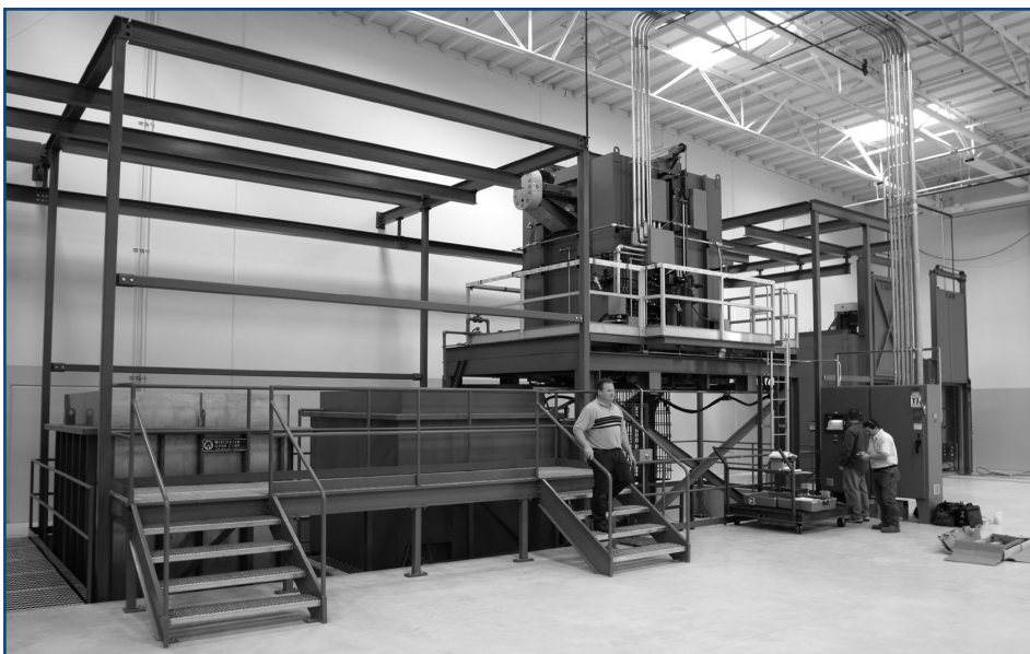
Custom built to RHC specifications, the aluminum heat treating furnace will allow RHC more control over part production.
